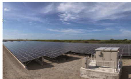
Sakata Mega Solar Power Plant (Sakata City, Yamagata)
